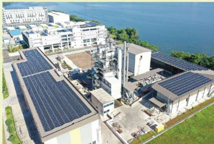
Rooftop Solar Panels
