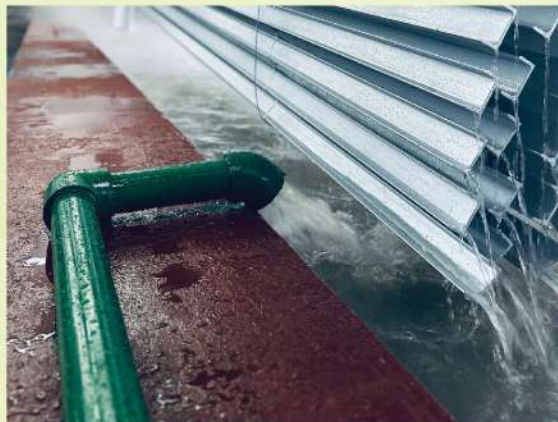
Quenching Water Tank Return Pipe Outlet in Operation
