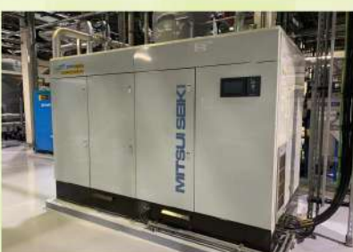
Photo of new air compressor with variable speed drive functionality
